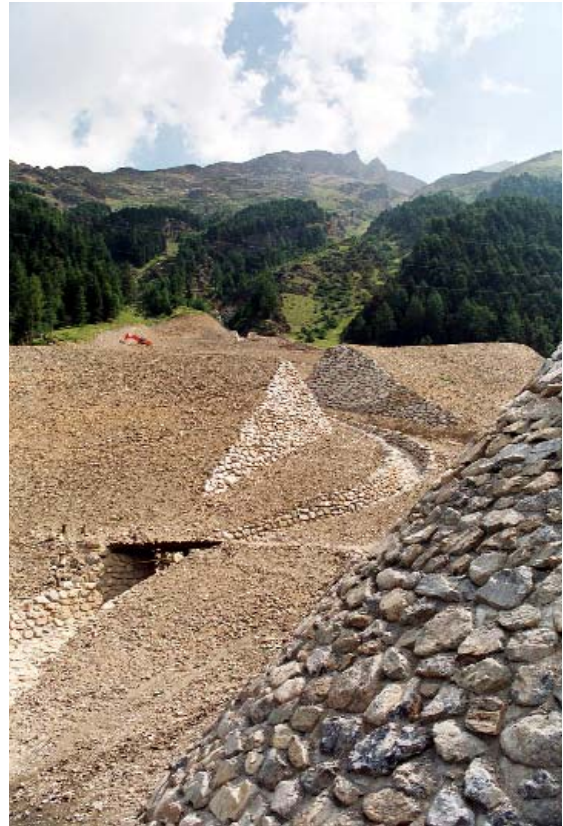
Debris flow protection works above Pontresina (Engadine)
